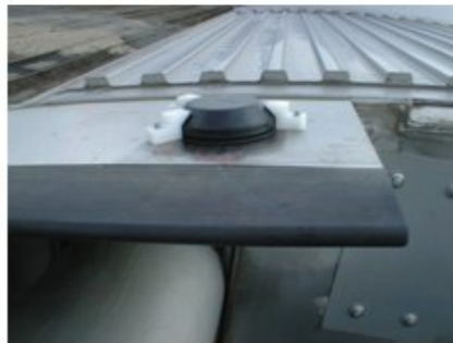
Roof-Mounted GPS Antenna
