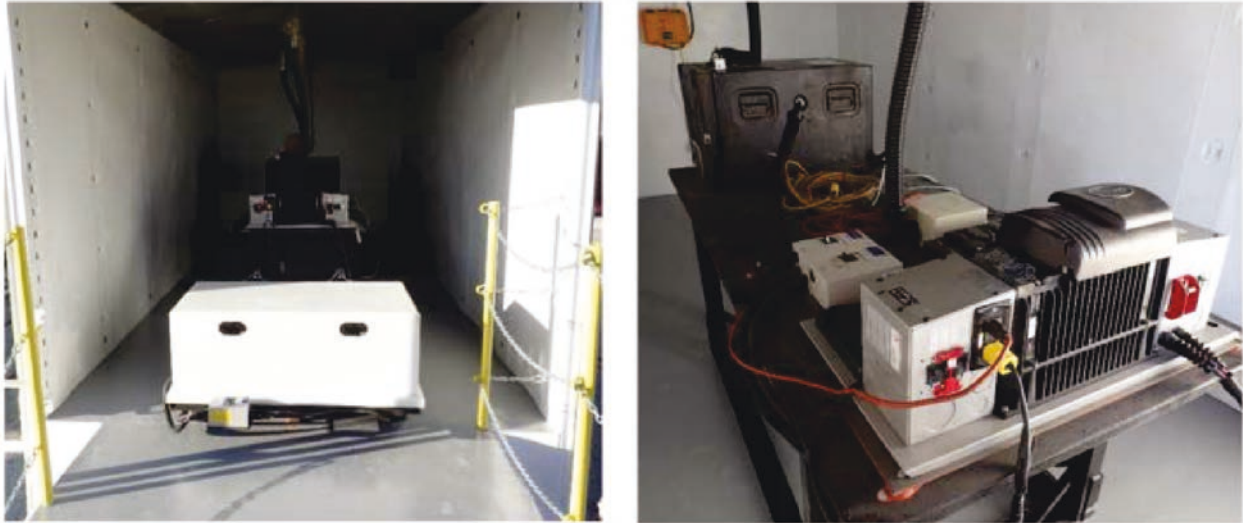
Figure 51: Freight ATGMS Power System Installation
