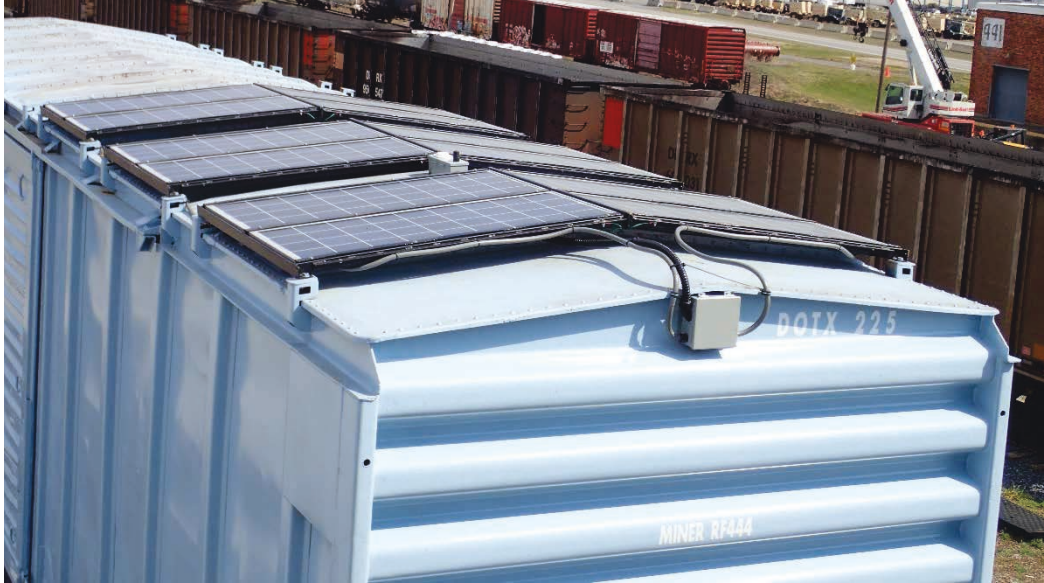
Figure 49: Roof-Mounted Equipment on DOTX 225
