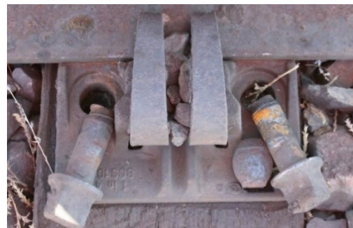
Figure 3. Broken lag screws in McKay fastening system
