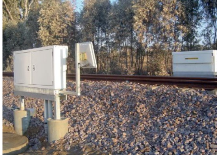
Figure 3-2. An example of RailBAM® detector installed on the track [24]
