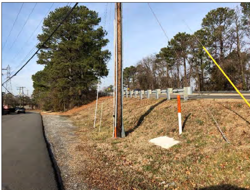
FIGURE 4-194: ROAD CONSTRUCTION AND BURIED UTILITY DISTURBANCE IN AREA 6C ALONG DUMBARTON ROAD, LOOKING WEST
