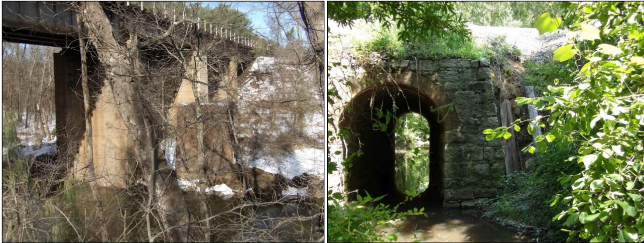
FIGURE 3-175: A RAILROAD BRIDGE OVER THE NORTH ANNA RIVER (042-0731), NORTH OBLIQUE (LEFT); A RAILROAD CULVERT OVER A STREAM NEAR LORTON MARKET ROAD (500-0001-0019), LOOKING EAST (RIGHT)
