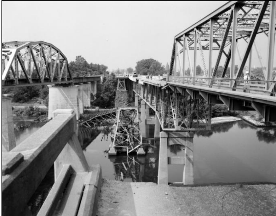
FIGURE 3-4: VIEW OF THE BRIDGE, CSXT TRACKS OVER OCCOQUAN RIVER ON THE LEFT OF THE IMAGE, LOOKING SOUTH, AFTER AGNES IN 1972 (LIBRARY OF VIRGINIA 1972B)
