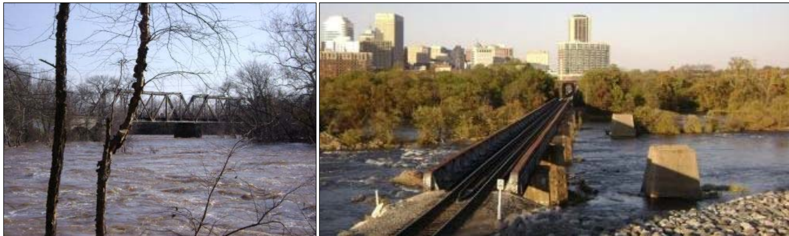
FIGURE 3-162: VIEW OF THE THROUGH TRUSS BRIDGE CARRYING THE SOUTHERN RAILWAY SEGMENT ACROSS THE JAMES RIVER, LOOKING SOUTHEAST (LEFT); VIEW OF THE JAMES RIVER BRIDGE CARRYING THE SOUTHERN RAILWAY SEGMENT, LOOKING NORTHEAST (RIGHT) (BRIDGEHUNTER.COM 2017C)
