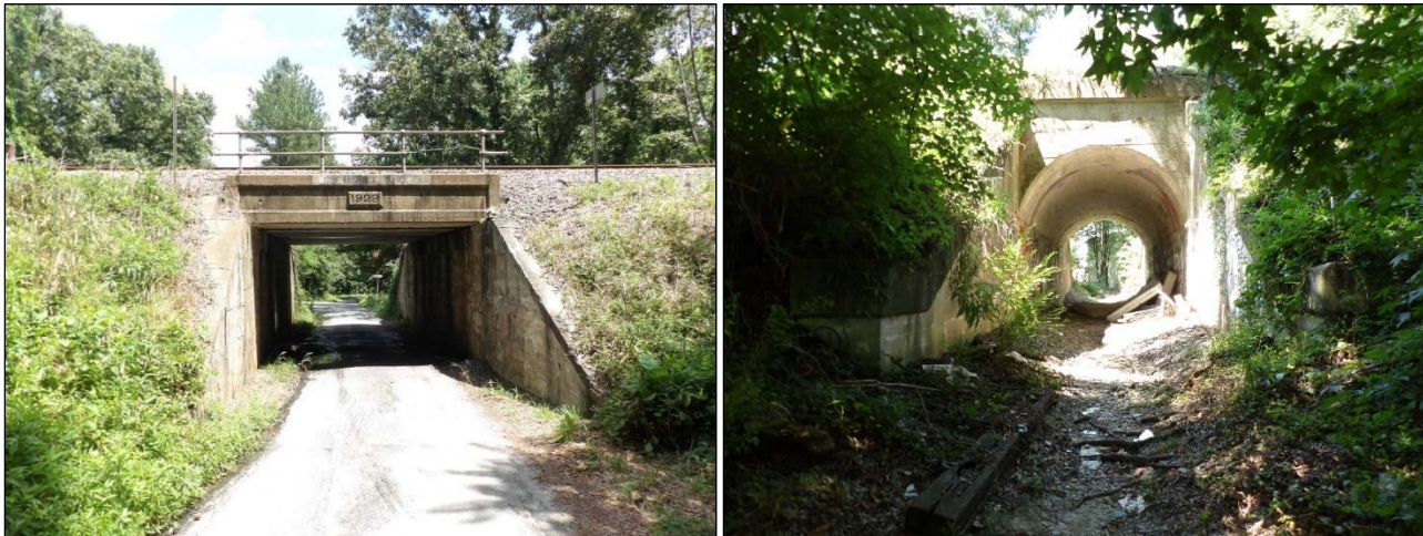
FIGURE 3-176: A RAILROAD CULVERT WEST OF DABNEY ROAD, USED TO ALLOW LIVESTOCK TO PASS (500-0001-0023), LOOKING WEST (LEFT); BRIDGE AT TAYLORSVILLE ROAD (042-5306), LOOKING EAST (RIGHT)
