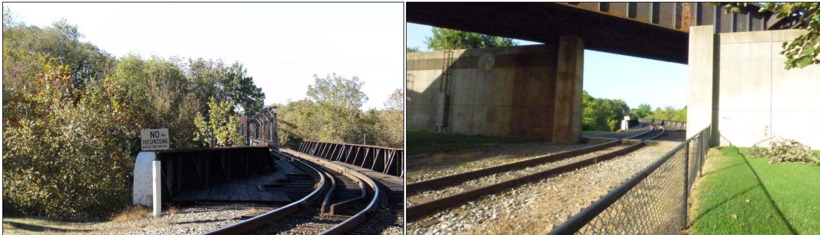
FIGURE 3-161: NORFOLK-SOUTHERN RAILROAD STEEL-PLATE PONY TRUSS BRIDGE IN RICHMOND, LOOKING SOUTHWEST TOWARD A THROUGH TRUSS (LEFT); VIEW OF SOUTHERN RAILWAY SEGMENT'S ONE TRACK, LOOKING SOUTHWEST (RIGHT)
