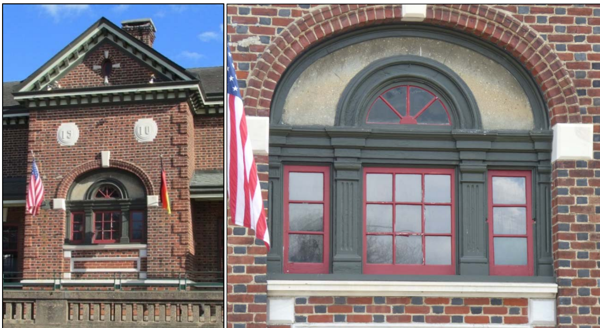
FIGURE 3-47: FREDERICKSBURG TRAIN STATION, DETAIL OF PROJECTING BAY AND PALLADIAN WINDOW ON NORTH ELEVATION
