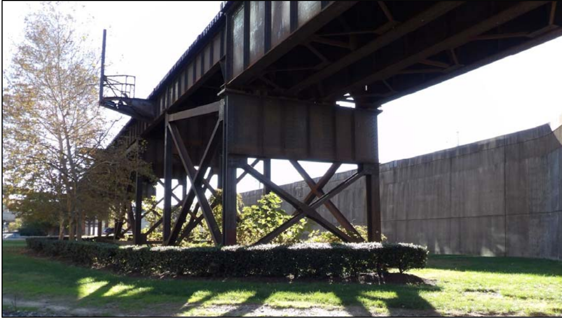
FIGURE 3-148: A C&O ELEVATED STEEL-PLATE-GIRDER BRIDGE AT SOUTH 14TH STREET, RICHMOND, VA, LOOKING SOUTHWEST
