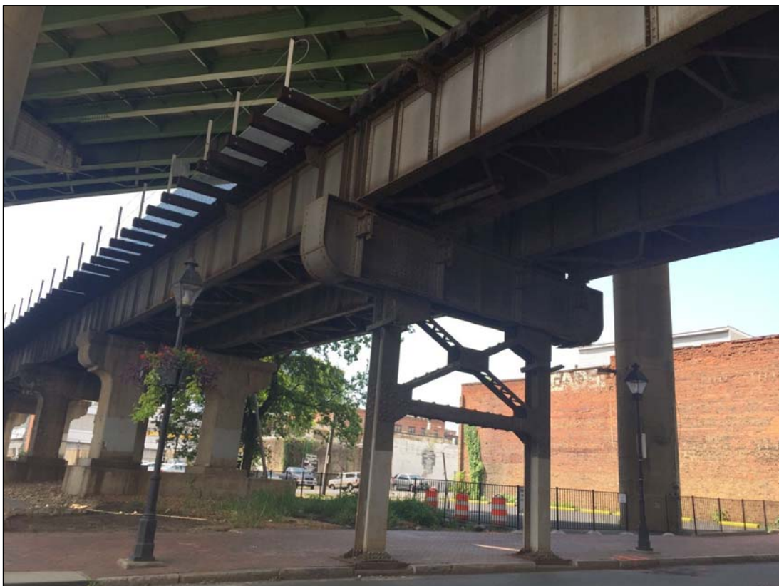
FIGURE 3-149: ELEVATED SUBSTRUCTURE OF THE RAIL LINE IN RICHMOND, LOOKING WEST FROM THE VIRGINIA CAPITAL TRAIL
