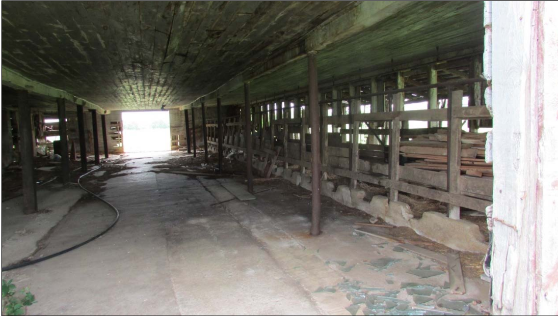
FIGURE 3-129: VIEW OF CENTRAL AISLE AND FEEDWAY AT RIGHT IN BARN LOOKING SOUTHEAST
