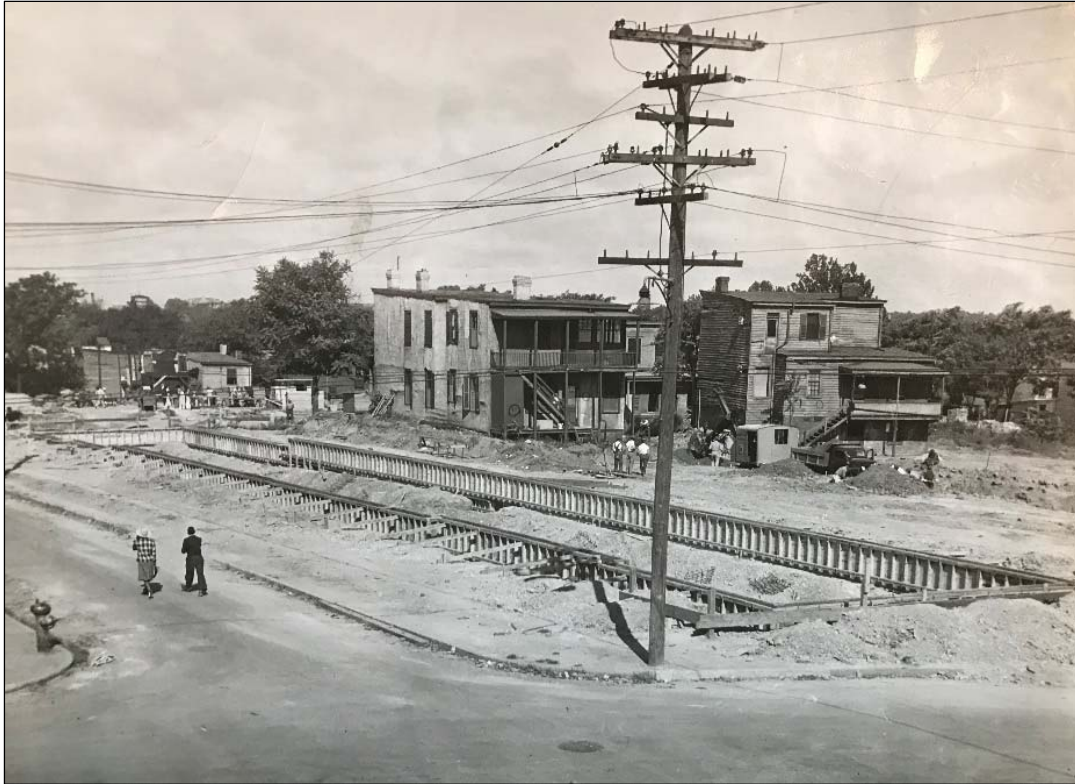
FIGURE 3-186: PHOTOGRAPH OF INITIAL CONSTRUCTION OF ONE OF THE APARTMENT BUILDINGS OF THE "GILPIN COURT SLUM-CLEARANCE PROJECT" (RRHA 1941)
