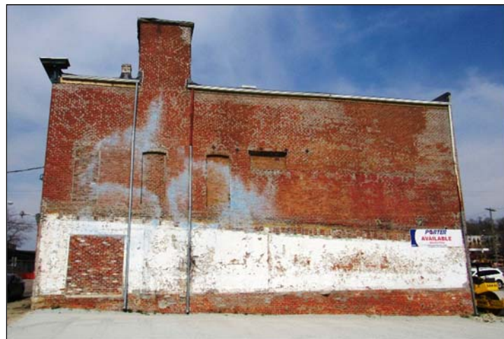
FIGURE 3-207: GHOSTING ON SOUTHWEST ELEVATION
