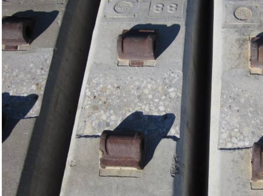
Figure 4. Detailed View of Ground Rail Seat with 0.1875-inch triangular RSD before installation at FAST
