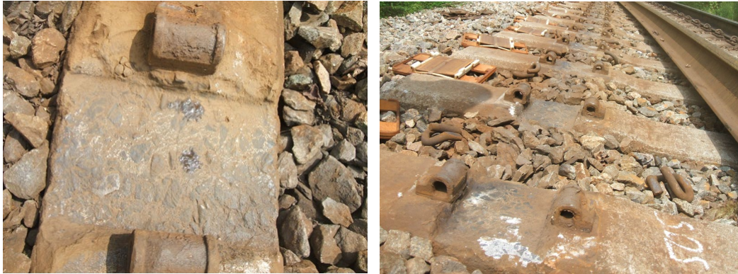
Figure 1. Rail Seat Deterioration
