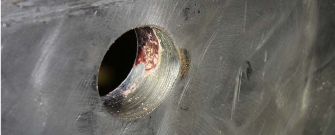
Figure 53. Plastic deformation of coupler pocket hole for shear bolt 3 (trailing end, toward rear of locomotive)
