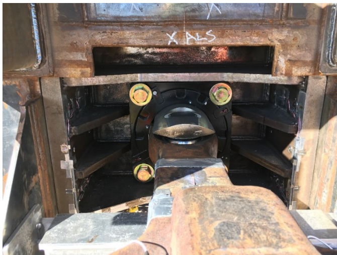
Figure 34. PBC installed within the sliding lug
