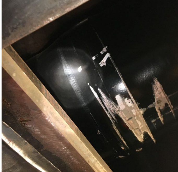
Figure 48. Cracked paint on the right side of the PBC deformation tube, indicating tube crush
