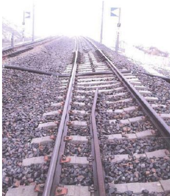
Figure 3.4 Guard rail protection (Abtahi, 2013)
