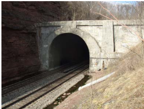
Sand Patch Tunnel Liner Notching
