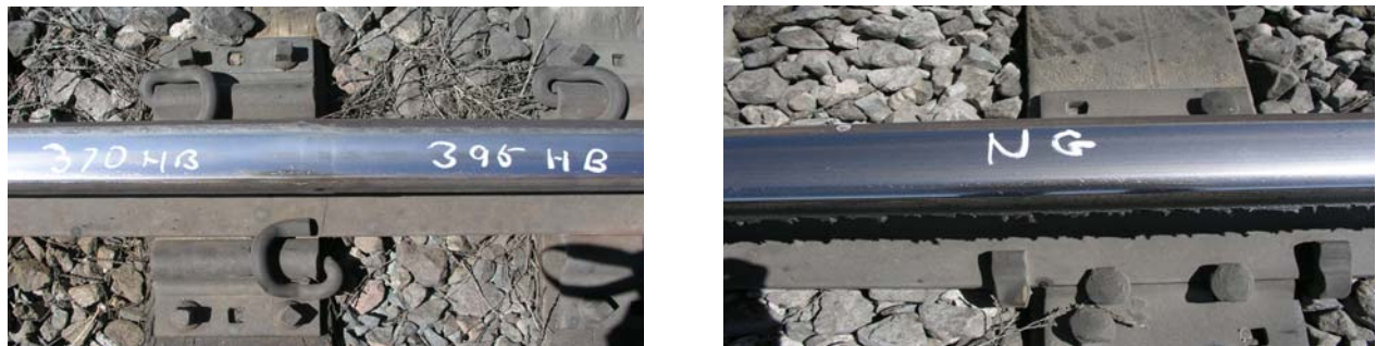
Figure 1. Condition of Unground Rails after 515 MGT Low Rail (left), High Rail (right)
