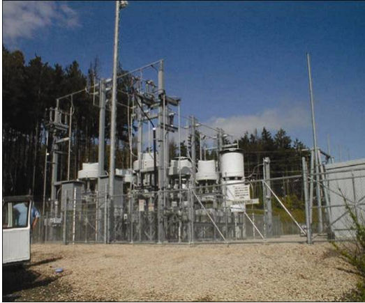
Figure 2-14 Traction power supply station
