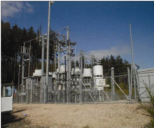
Figure 2-14 Traction power substation
