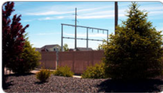
Figure 3.16-65 Example of Power Substation in Urban Setting, with Landscape Screening and Fence
