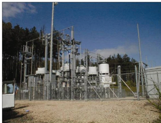
Figure 2-15 Traction Power Substation
