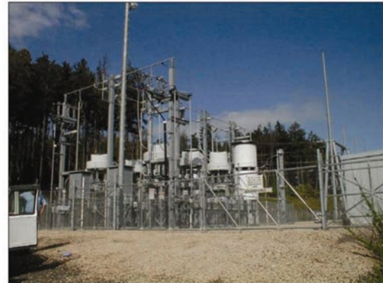
Figure 2-15 Traction Power Substation
