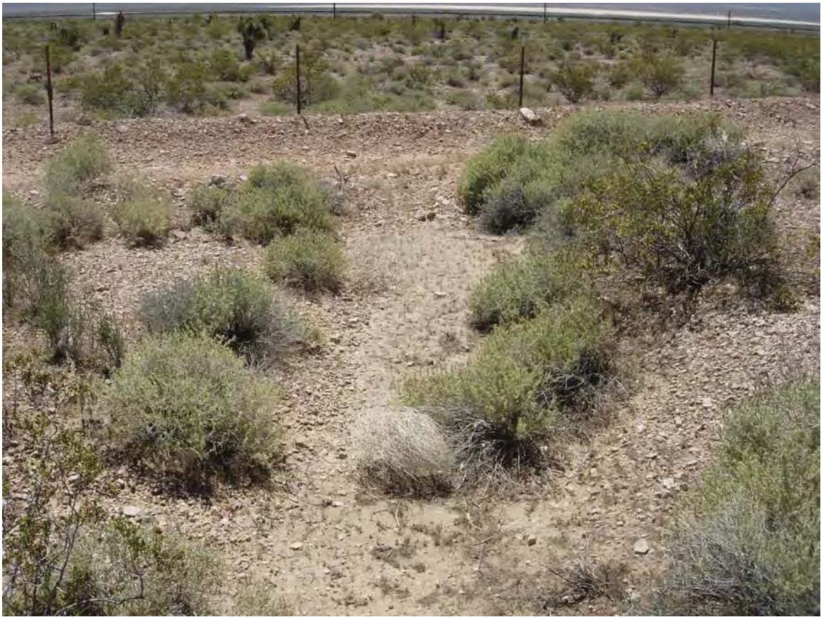
Exhibit A. Figure 39. Manmade drainage connecting to road culvert within HUC 8 Ivanpah-Pahrump Valleys / HUC 12 160600151401-Frontal Jean Lake Subwatershed
