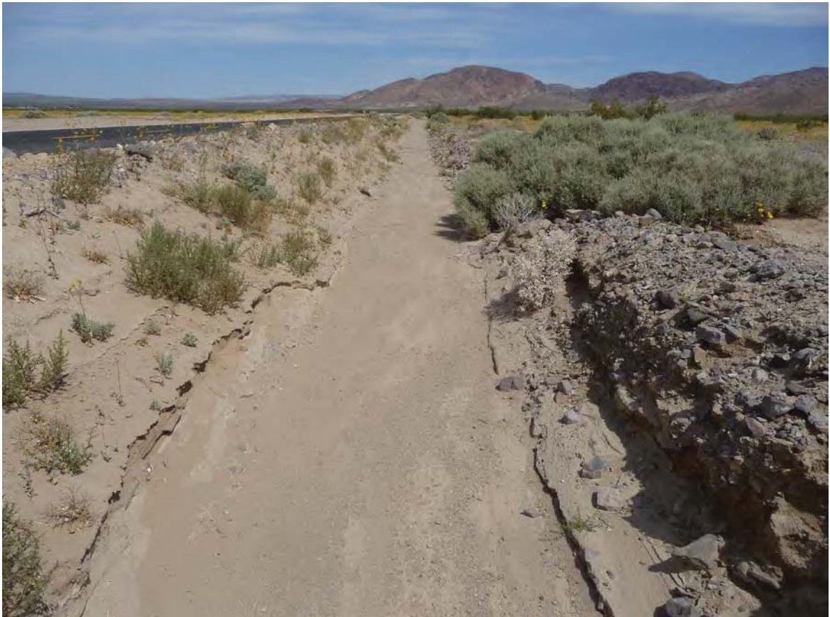
Exhibit A. Figure 24. Manmade drainage connecting to ephemeral drainage within HUC 8 Mojave / Coyote-Cuddeback Lakes Watersheds / HUC 12 Odessa Canyon Subwatershed
