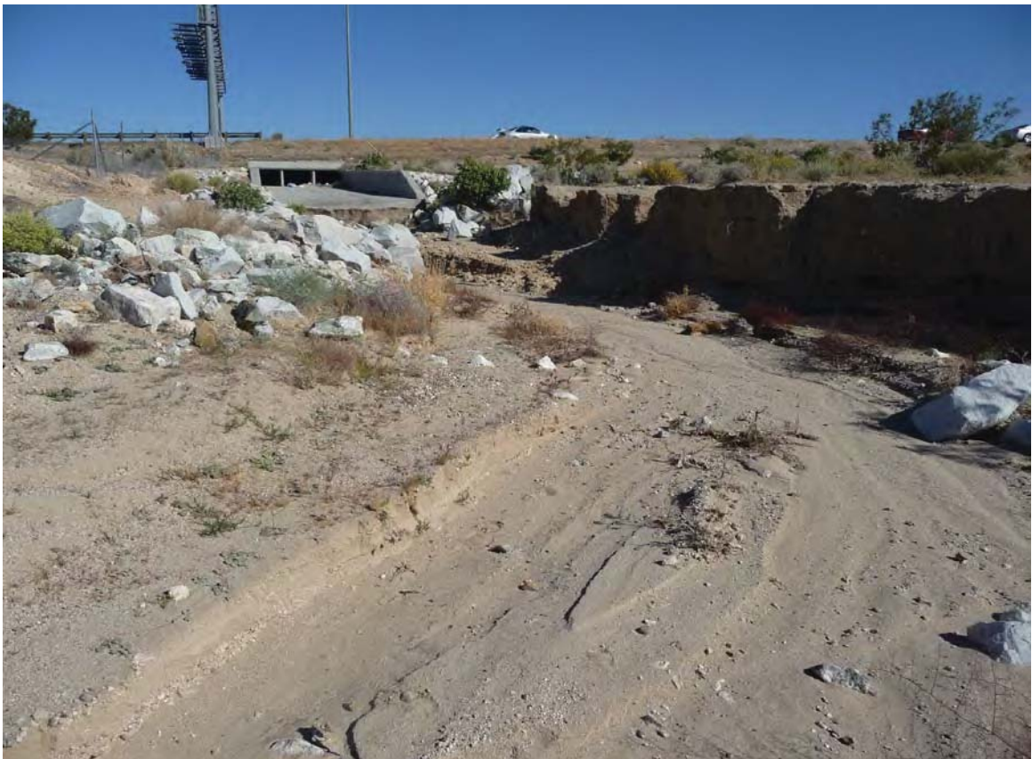
Exhibit A. Figure 18. Manmade drainage connecting to road culvert within HUC 8 Mojave / Coyote-Cuddeback Lakes Watersheds / HUC 12 Town of Lenwood-Mojave River Subwatershed
