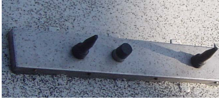
Hardware Corrosion Figure 12a
