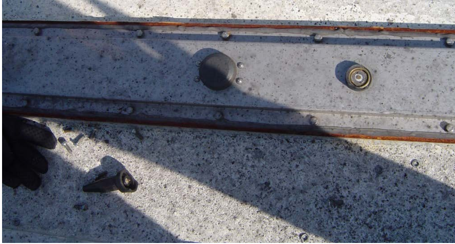
Plate Corrosion Broken Antennas Figure 12
