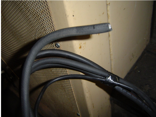
Un-Terminated Cables Figure 11
