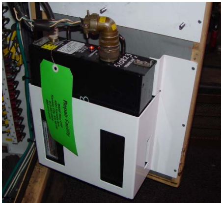
HOT/EOT Transmitter Figure 9
