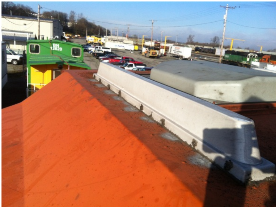
STI-CO HDLP-MB-PLLG25-BN Installed Figure 4
