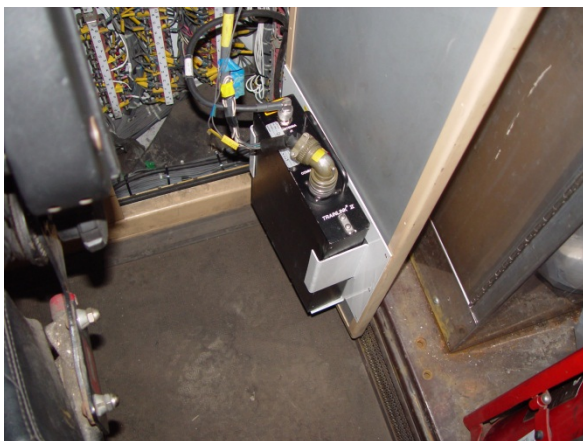
HOT/EOT Transmitter Figure 13
