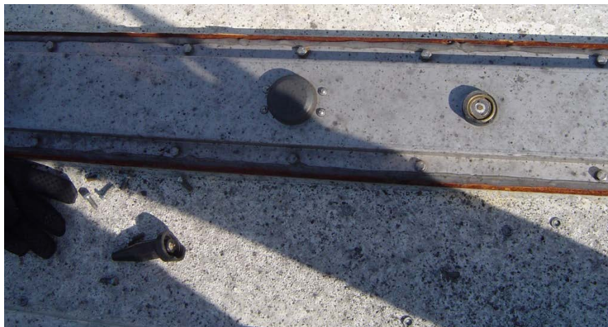
Plate Corrosion Broken Antennas Figure 12
