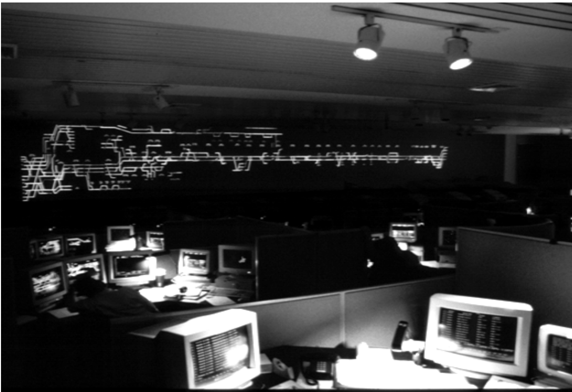
Figure 2. Dispatch Center 1. The Wall Panel Overview Schematic is Projected at the Front of the Room.
