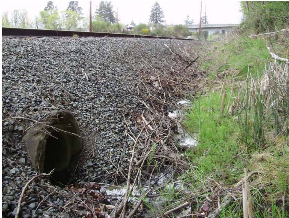
Photo 6. Wetland C. Culvert through which water flows out of wetland and under BNSF rail. Facing northwest (2011).
