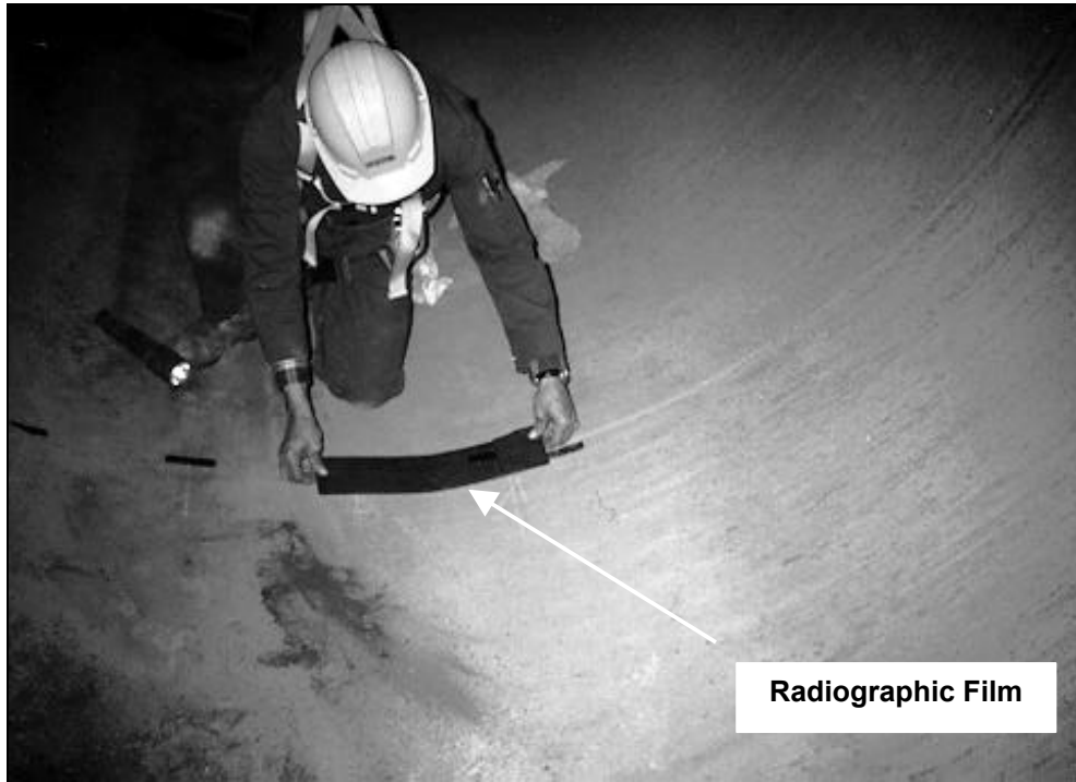
Figure 36. Film Placement at the Transverse Butt Weld in the Interior of the Tank for Radiographic Inspection
