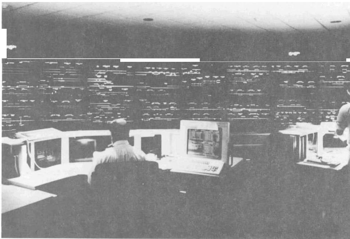
Figure 2.3-1: View of a Small Portion of CSX Operations Control Room Showing Work Stations of Chief Dispatchers and Power Coordinators.
