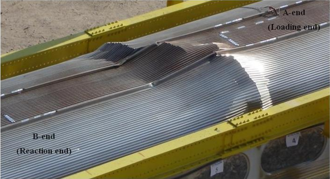
Figure 28. Crippling on Roof – Side View
