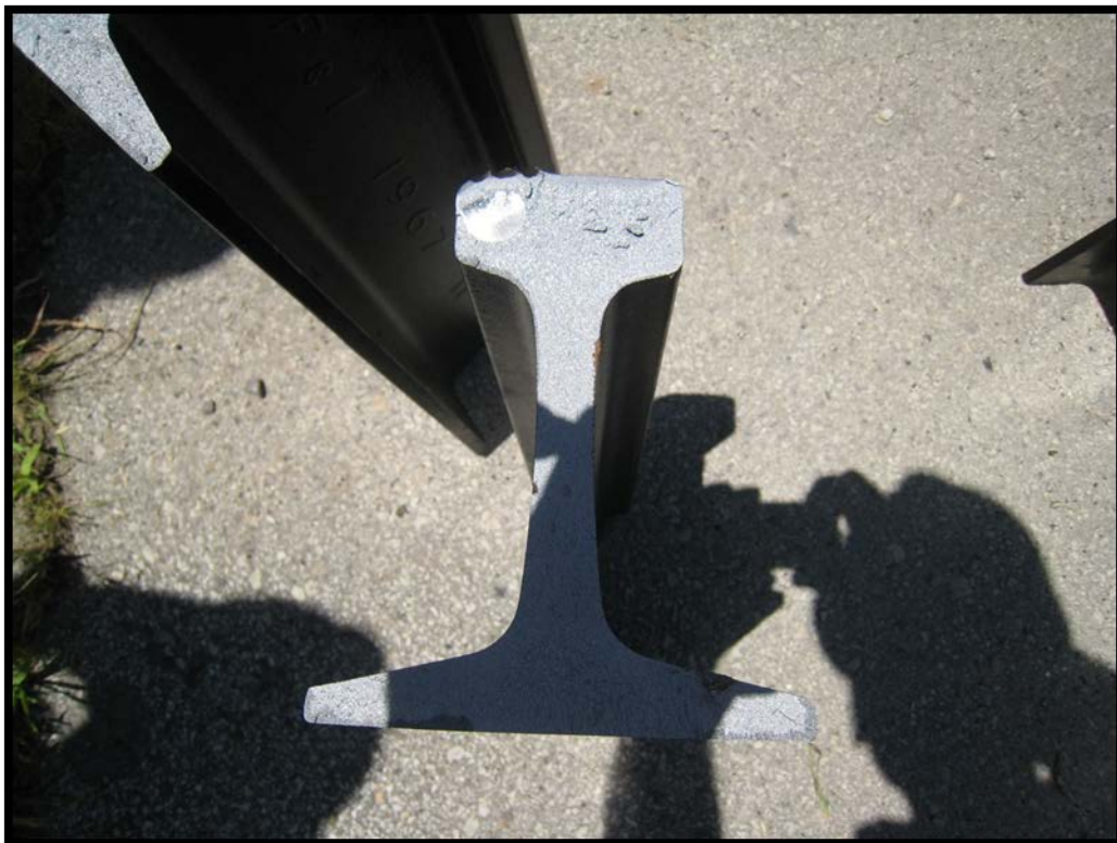
Figure 3.1. A picture of a Transverse Defect at the gage corner of the railhead.
