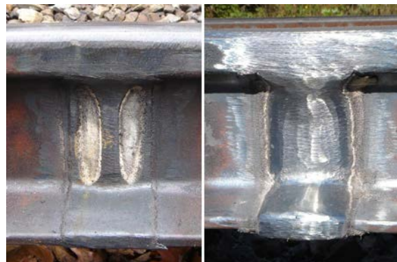
Figure 1. WGWs—Railtech Boutet (left); Orgo-Thermit (right)
