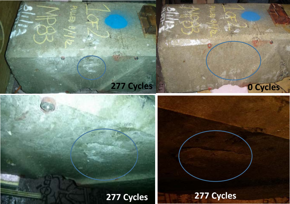
Figure 25: Tie #1-4397-F shallow cracking.
