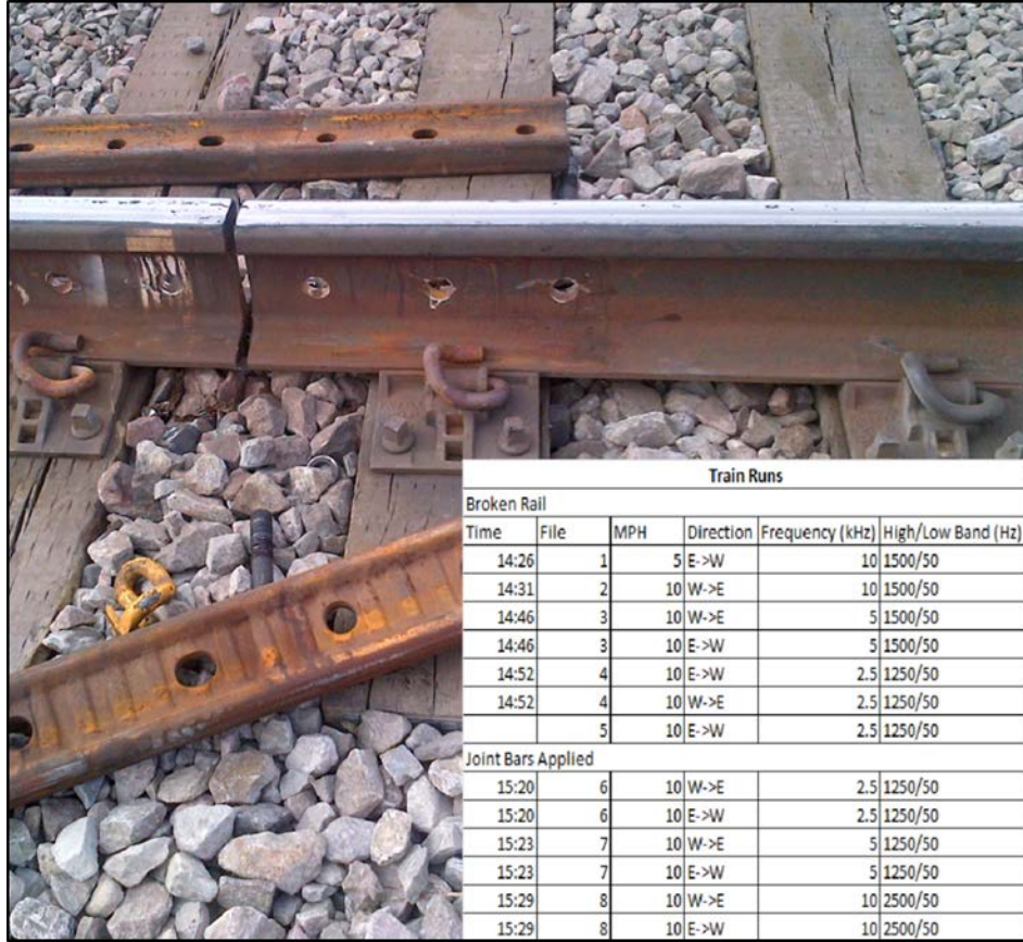
Figure 9: Light Locomotive Broken Rail Test
