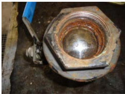
Valve body corrosion
