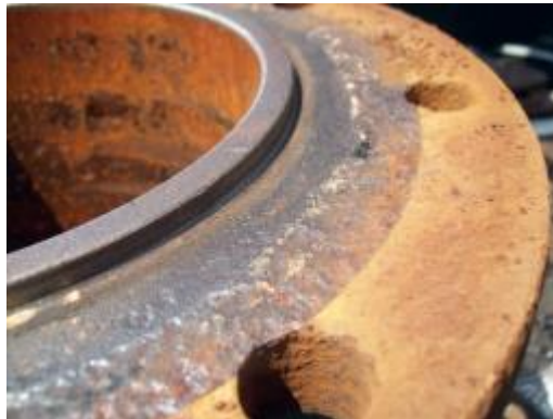
Corrosion of flange
