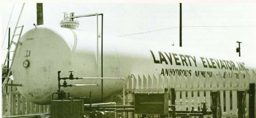
This is the largest of three anhydrous ammonia storage plants operated by Lavery Elevator, Inc. of Indianola, Iowa. Transport riser is at right. Single nurse tank loading riser is at left. All controls are in locked cabinets.
