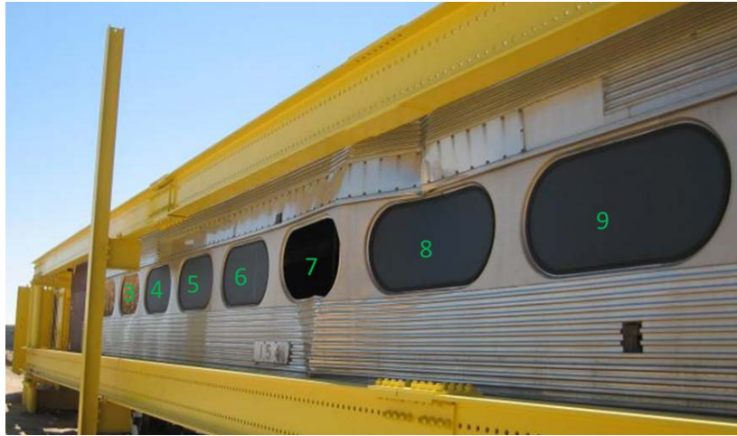
Figure 51. Damage to Left Sidewall, Car 248
