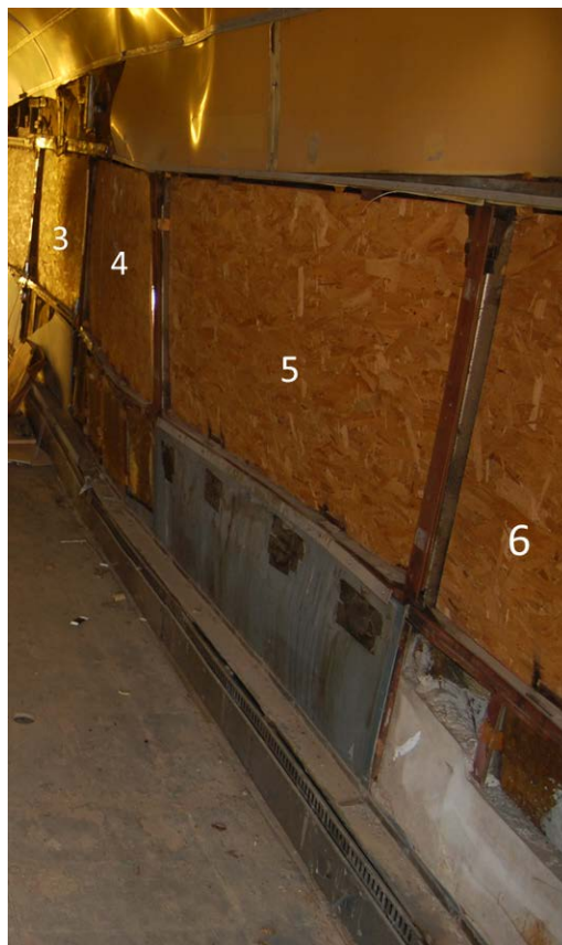
Figure 63. Damage to Right Side Interior of Car 244
