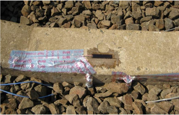
Figure 6.5. Concrete strain gage mounted to the center of a tie
