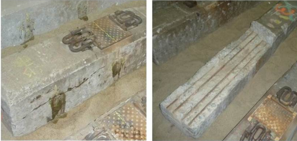
Figure 2.2. Photographs of the predominant mode of concrete tie cracking we investigated in this study; the crack on the left is revealed by alcohol.
