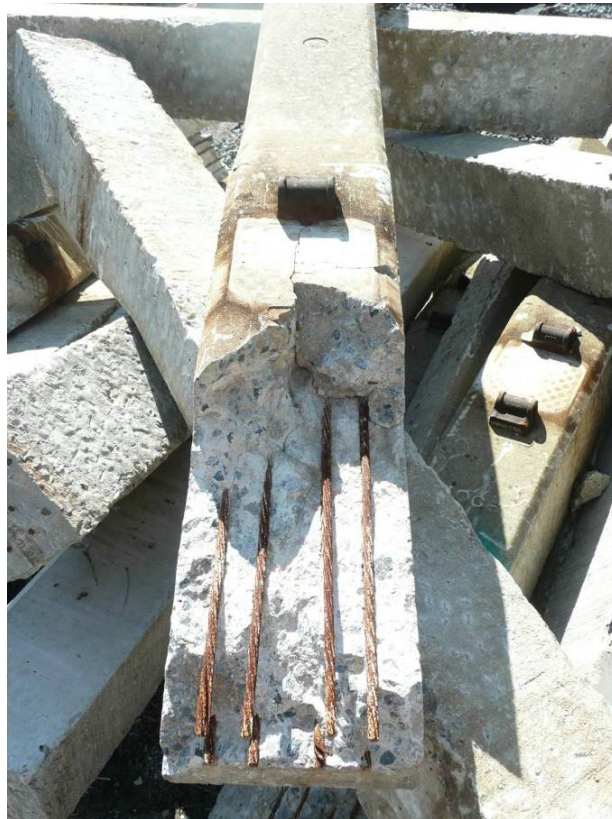
Figure 3.4. An example of a severely cracked tie from the MBTA Old Colony Line.
