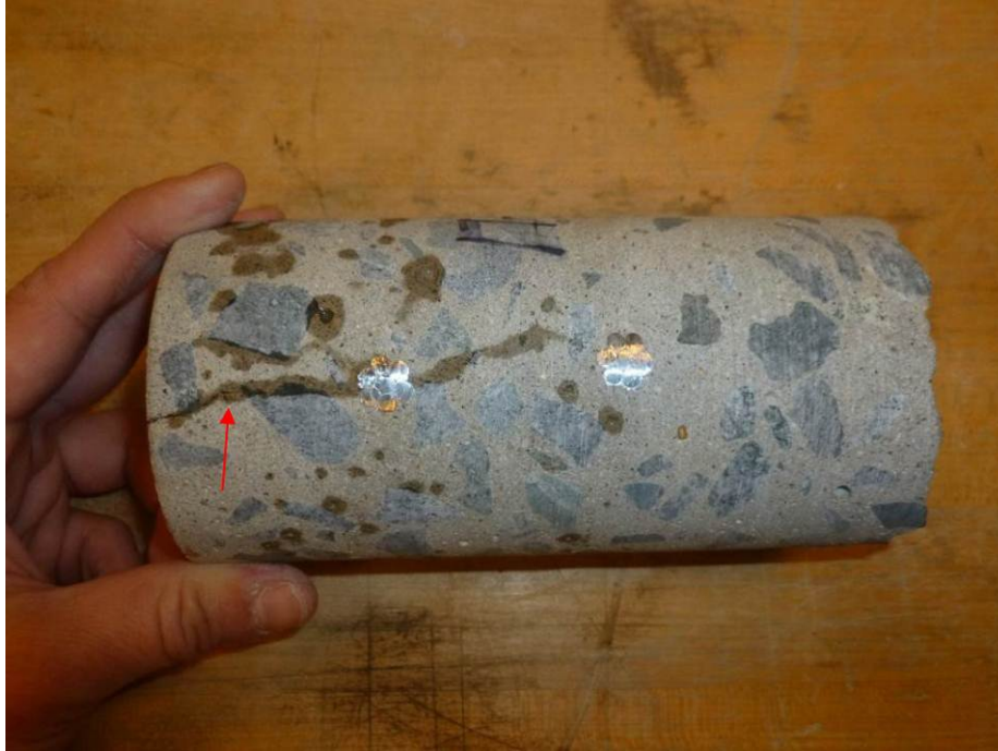
Figure 4.11. Core C17-3- sprayed with alcohol showing the lateral crack on the exterior surface extending into the concrete body and stopping at the second tendon.
