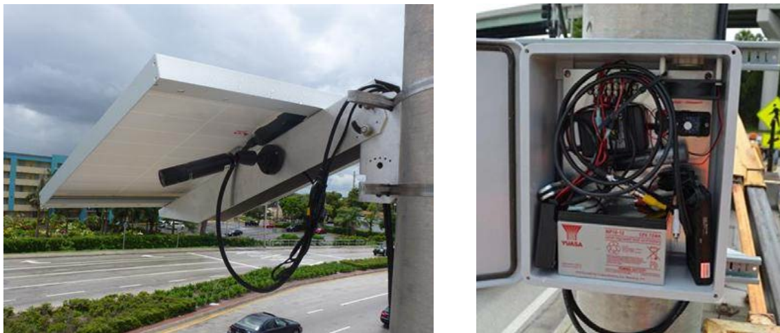
Figure 12. Camera and Solar Panel (left) and Utility Box (right)
