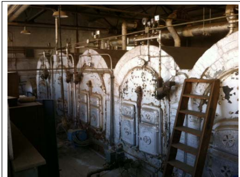
Photo No. 9. View of the interior of boiler room (note the original boilers in place; Photograph taken on 9/28/2011).
