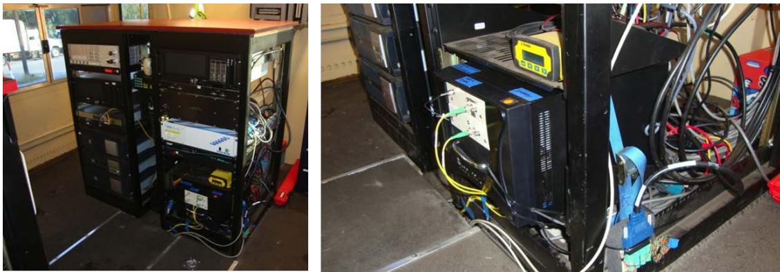
Figure 23: LIDAR computer installed onboard the track geometry car and linked to KVM system
