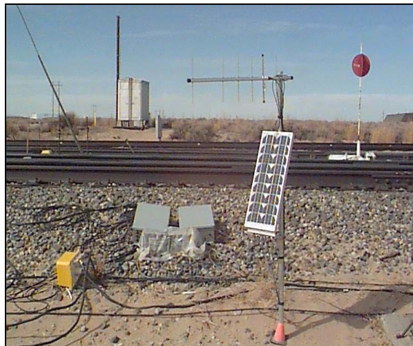
Figure 3. System 1 Solar Panel, Antenna, and Control Boxes
