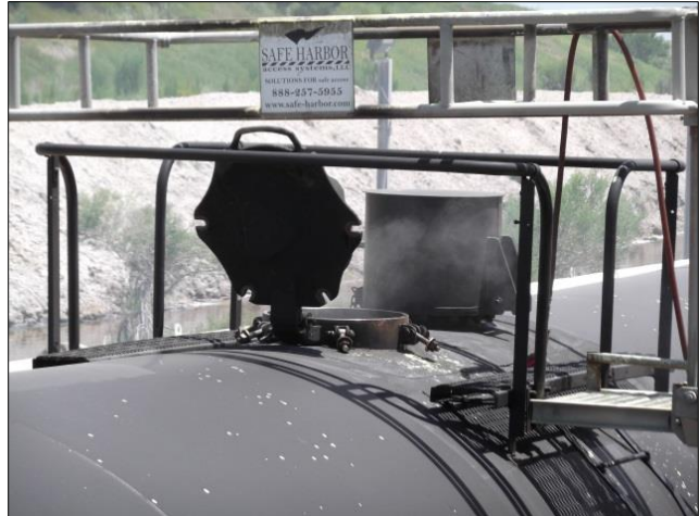
Figure 12: Open Dome Lid (Venting)
