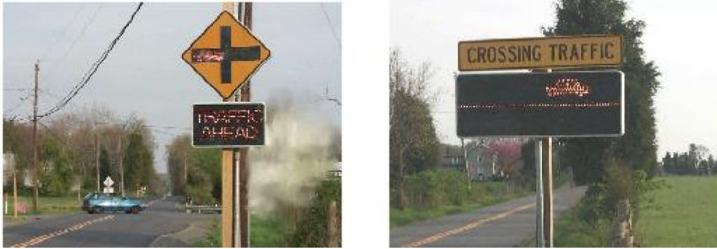
Figure 14. Collision warning signs for the major leg (left) and minor leg (right) of the intersection
