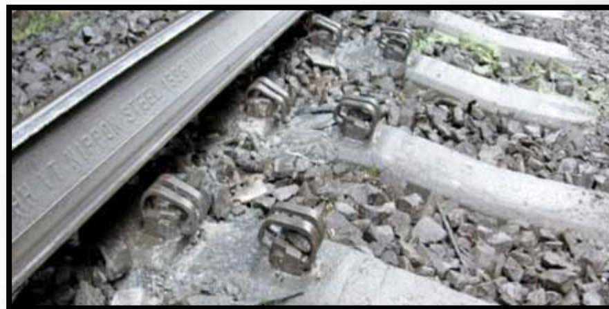
Rail Seat Deterioration in Concrete Ties
