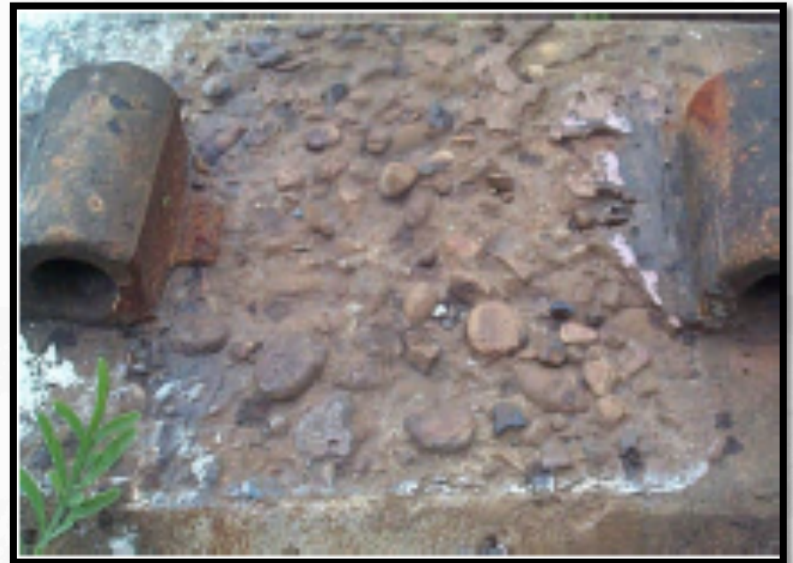
Abrasion due to Water Intrusion
